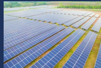
Xayaburi Power Plant
